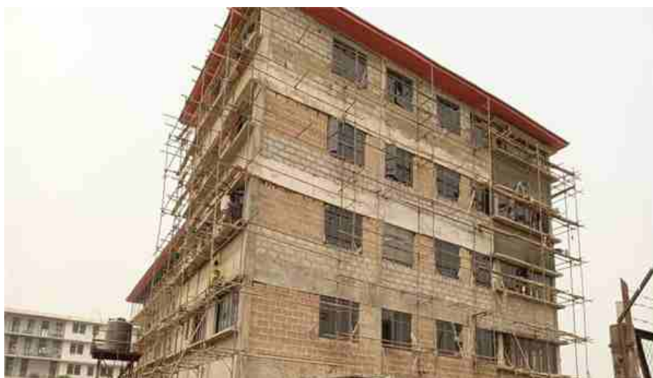
Ongoing Extension work on the Accident and Emergency Ward at UCH, Ibadan
