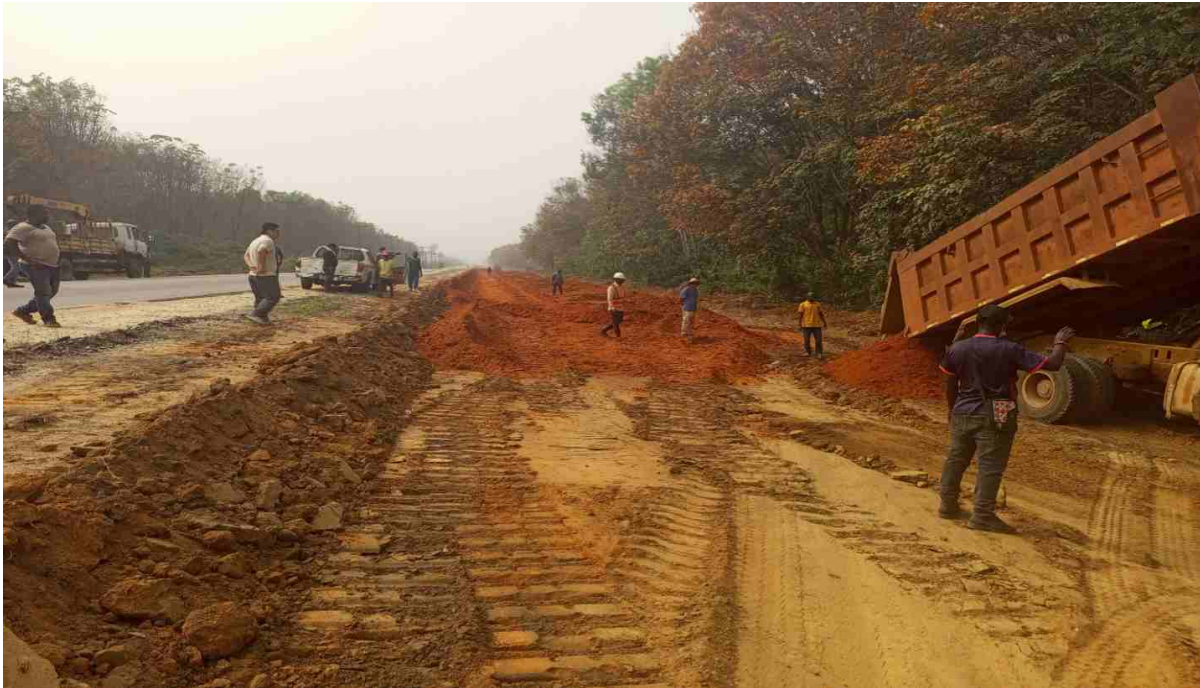
Earthworks Part of Section I of the dualization of Sapele - Agbor Road in Delta State
