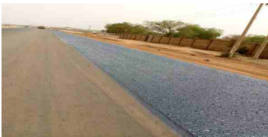
Laying of bituminous emulsion and spraying of aggregates for the second coat surface Kano Western By – Pass Road
