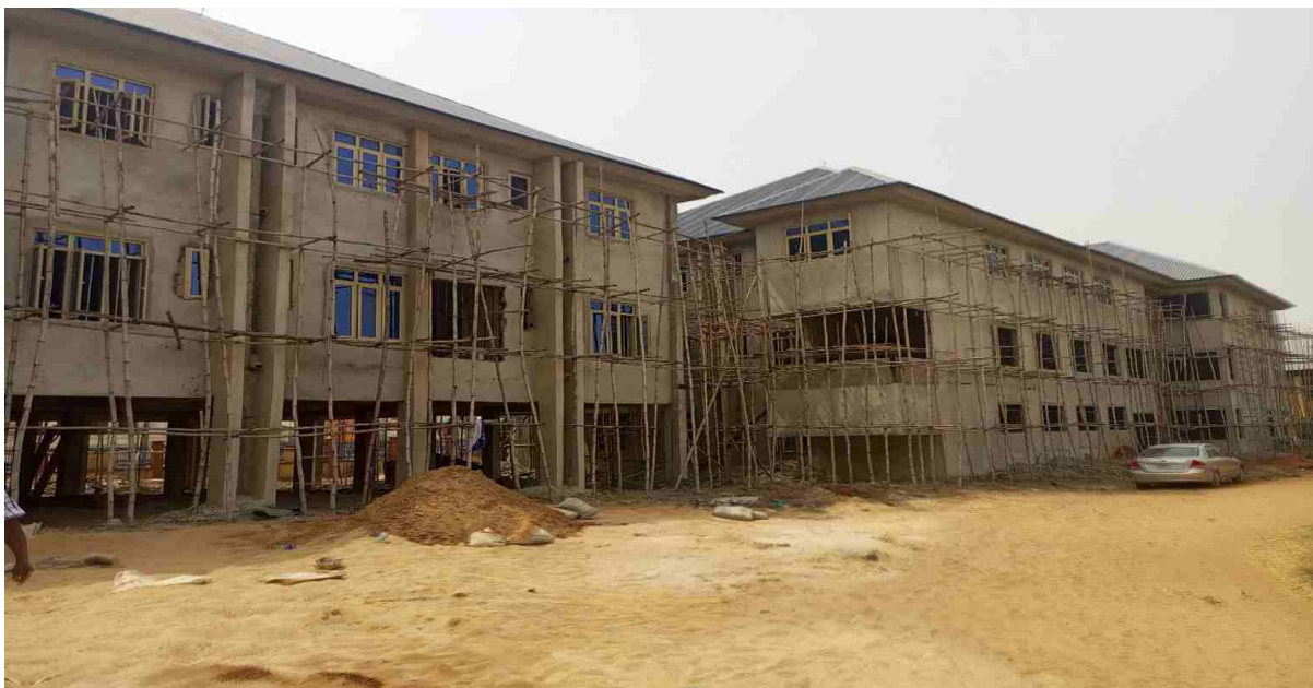
On-going Construction and Completion of Two-Story Sub-Specialty Complex at FMC, Asaba, Delta State
