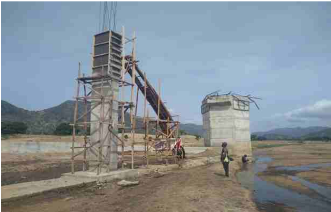
Intake Tower and Access Bridge under Construction at the Monkin Earth dam project in Taraba state
