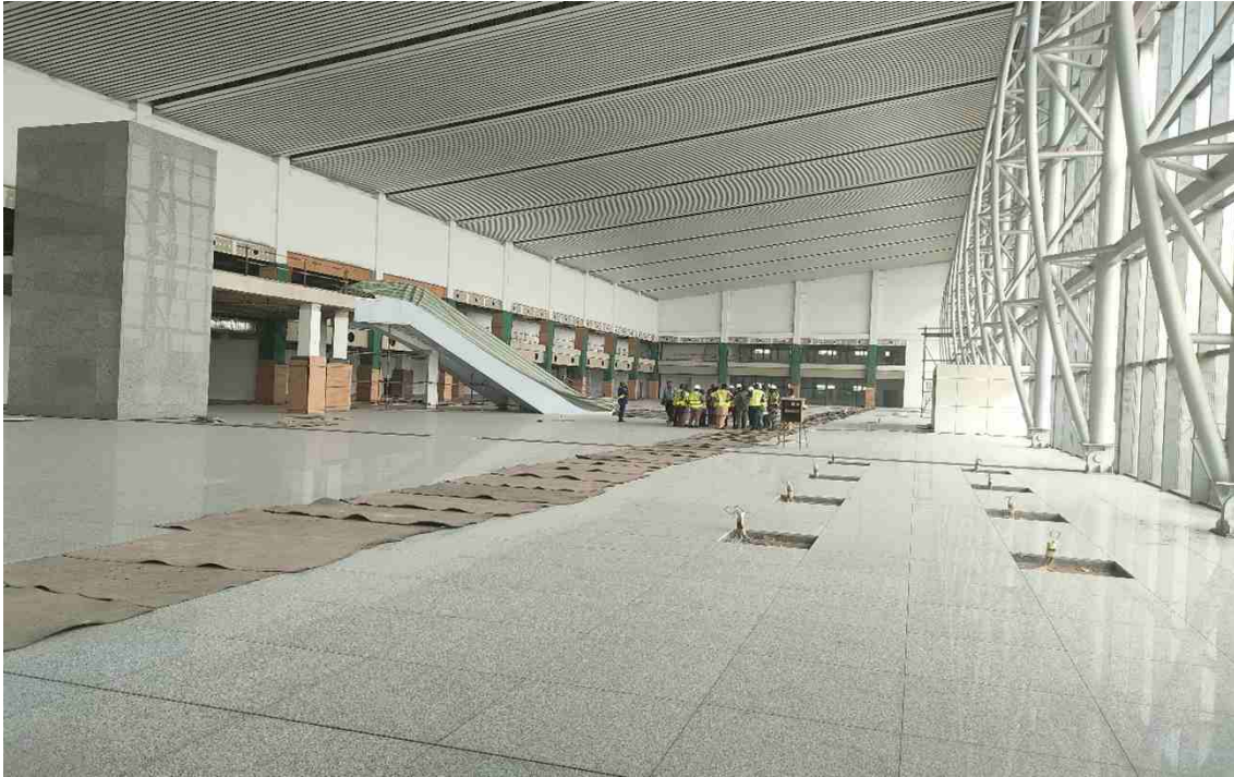
The view of the completed tiling of the international waiting Lounge at the Akanu-Obia international airport, Enugu
