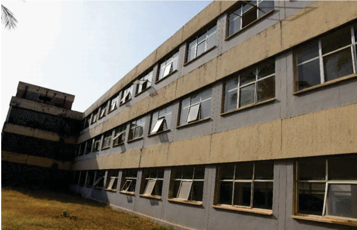
Fig. 32 Renovated Block D (female Students Hostel) at National Eye Centre, Kaduna State
