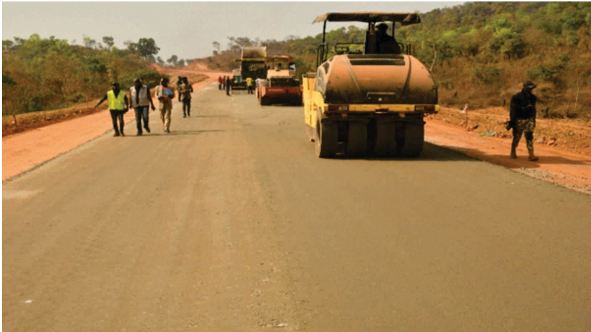
Fig.2 View showing 150mm thick crushed stone base course of Iluke – Ayetorokiri- Abugi- eggan road in kogi State
