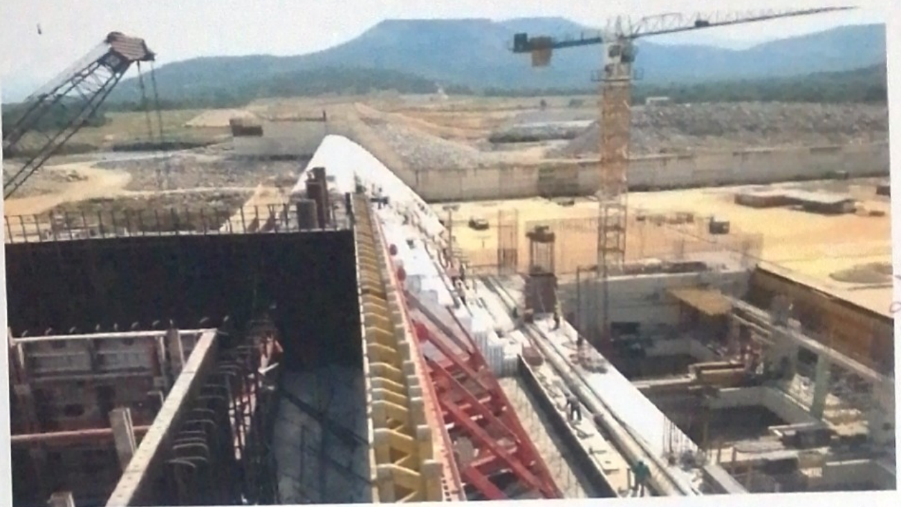
Section view of the spillway HP Station & Intake sections under construction at the Kashimbila/Gamovo Multi-Purpose Dam, Taraba State
