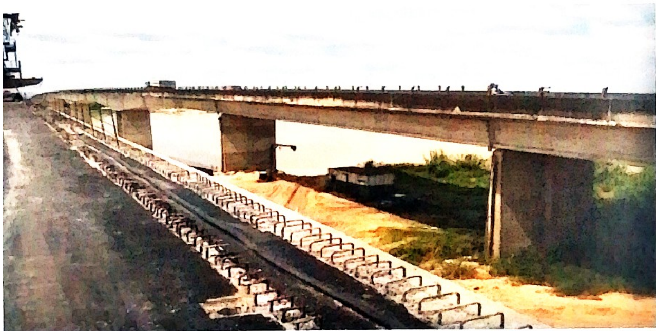
The Patani Bridge under construction – part of the Warri - Kaiama Road Project (East-West Road, Section I)
