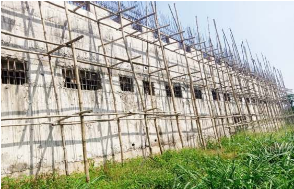
Side view of the on-going construction of one storey maximum Concrete Cell Block at Ogwashiuku Custodial Centre, Delta State
