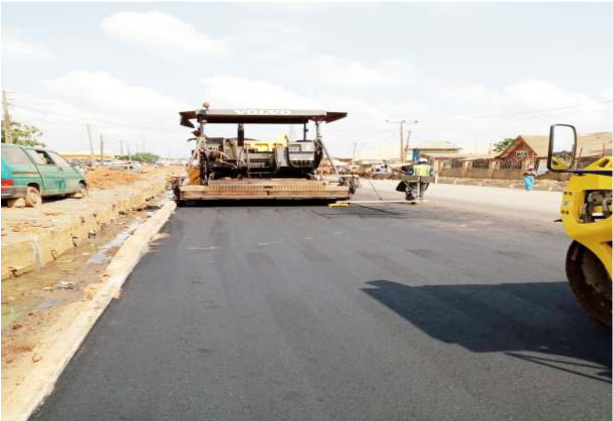
Asphalted Section of Rehabilitation of Ikorodu - Shagamu Road in Lagos / Ogun States.
