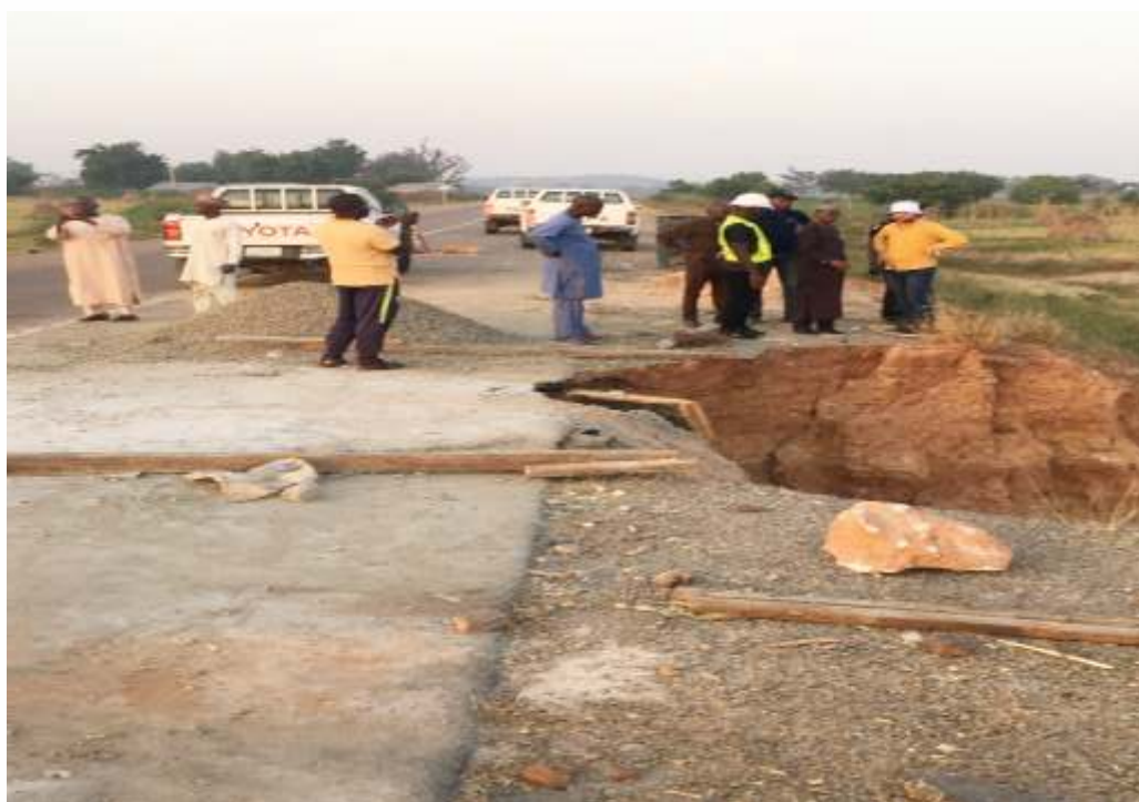
Bad portion of the completed Tumu-Pindiga Kashere (Gombe State) - Futuk Yola (Bauchi State) road
