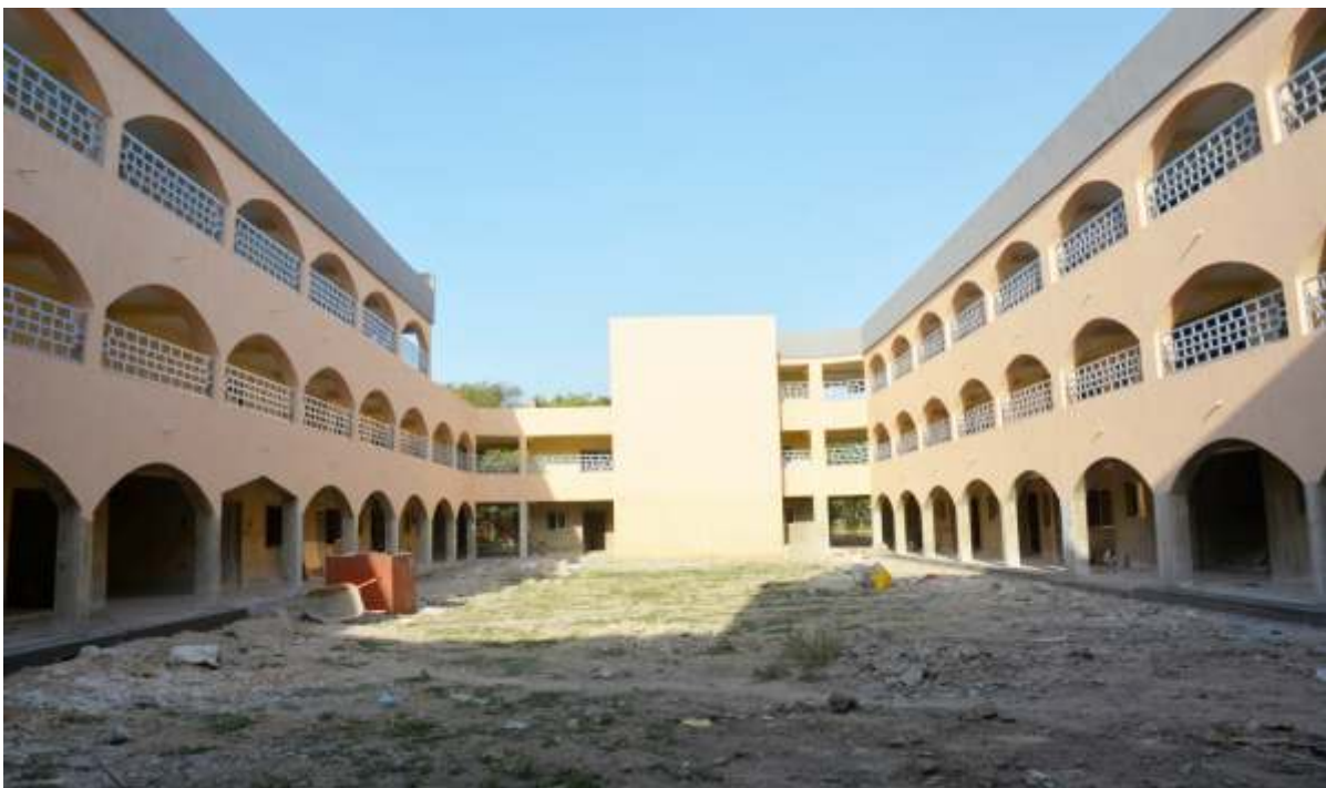
Inside view ongoing construction of 40 flats for Residents Doctors at AKTH, Kano
