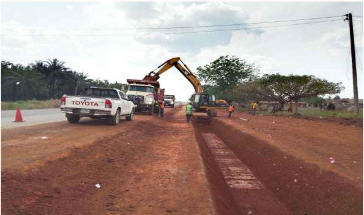
Ongoing construction of drainage along the 22km length asphalt on Makurdi-Naka-Adoka road in Benue State
