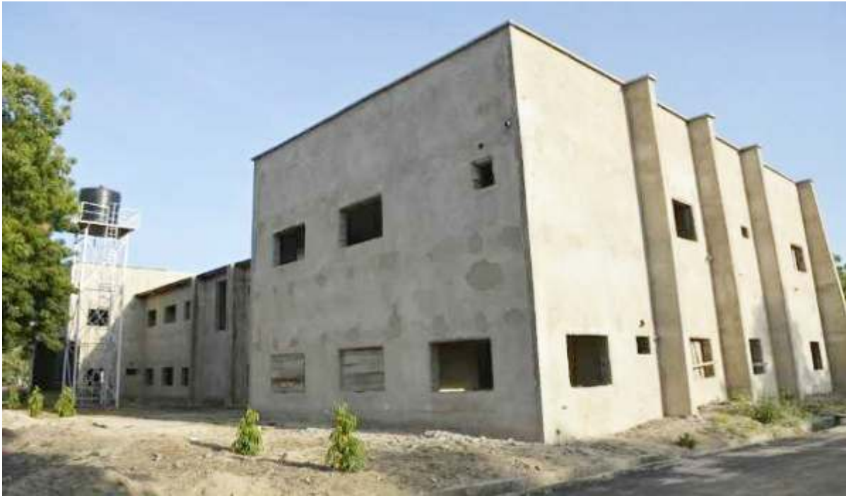
Ongoing construction of 2nos. Lecture Theatres for School of Post Basic Mid-Wifery at FMC, Birnin Kudu, Jigawa State.
