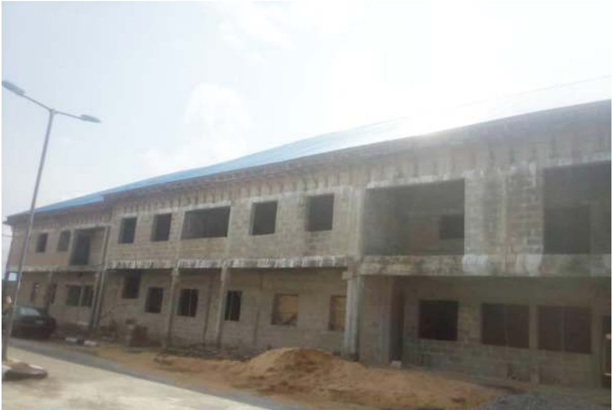
View of the theatre building showing roofing already completed at FMC Yenagoa, Bayelsa State
